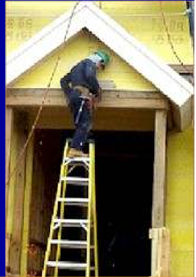
Improper use of the top rung of a step ladder
