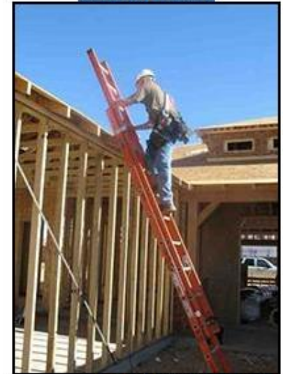
Ladder at Proper Angle Secured Footing
