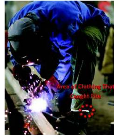
Figure 2. Site of Contact on Welder's Exposed Synthetic Clothing
