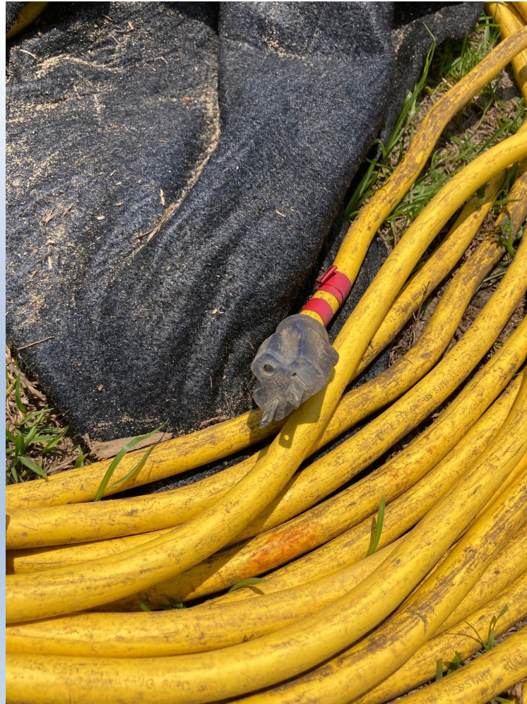
Missing Ground Pin
