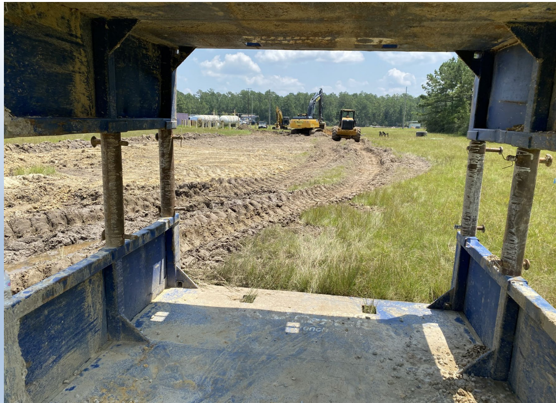
Trench box missing safety pins.
