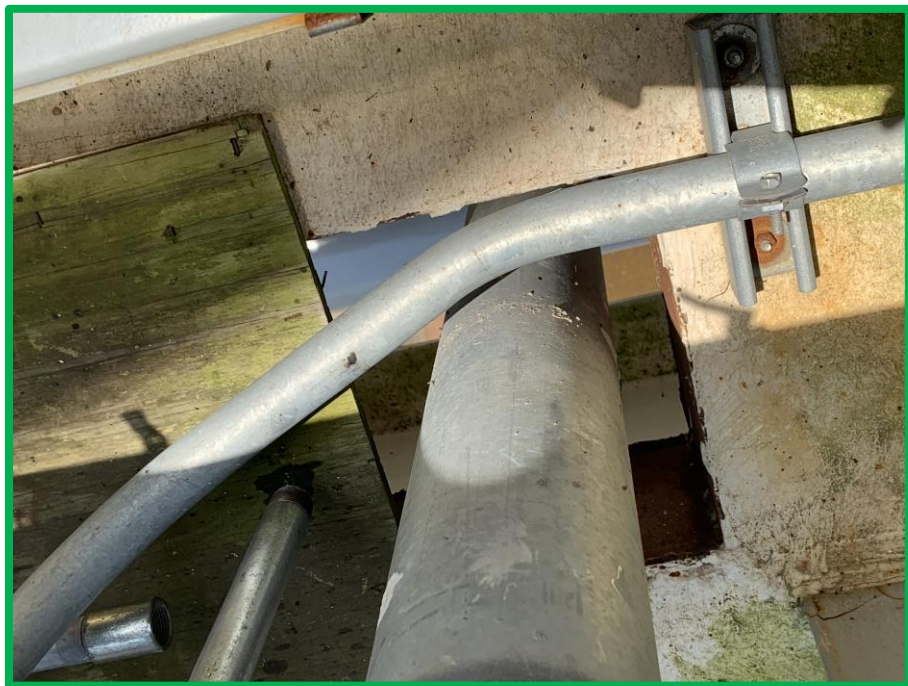
Before – Items can fall to lower level
