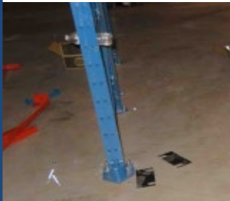
Leveling shims near metal upright where workers were installing racks.
