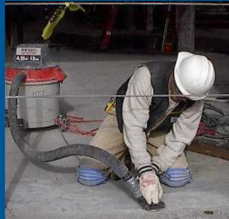
Concrete sander with exhaust ventilation
